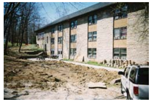
The new south patio and outside access to the dining room, with new sidewalk leading back to the parking lot.
